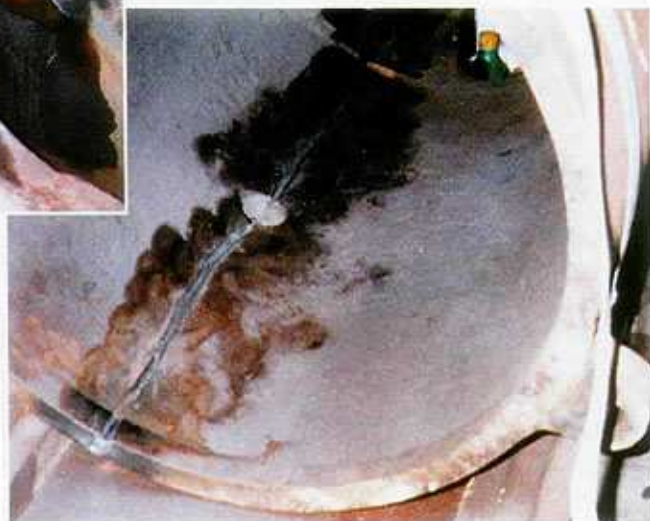
Below: Freeze crack ran the entire length of the cylinder water jacket.
